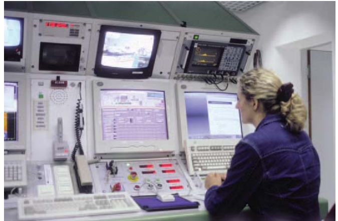
Fig.31: View of the control desk in the therapy control room TKR with the main control monitor in the center.
