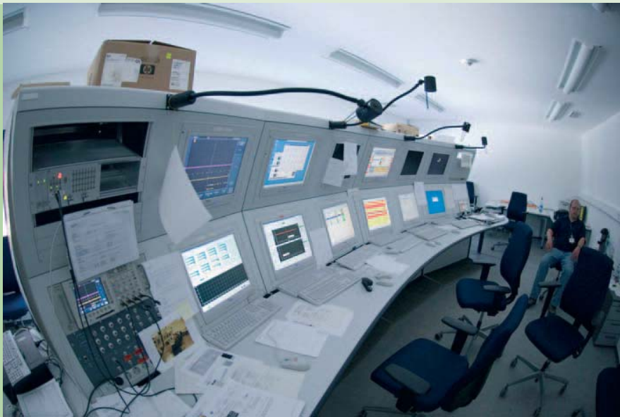
Control panel of the HIT facility.
