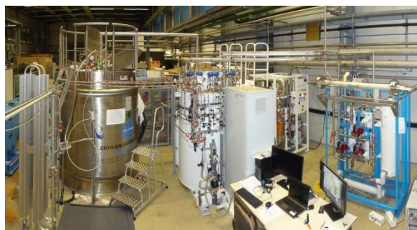
Figure 1: The HeSu plant. From right to left: purifier cold box and LHe storage
