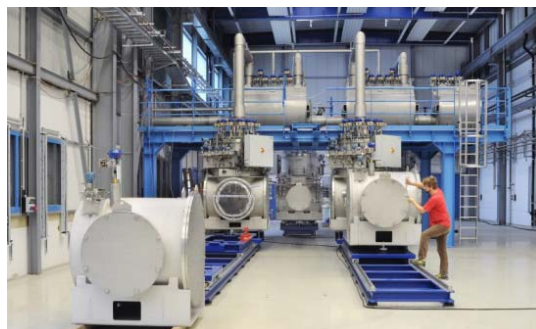
Figure 2: Ground floor: The two right-hand test benches. First floor: The two distribution boxes and the multi-purpose terminal.
