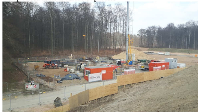
Figure 4: FAIR transformer field north
