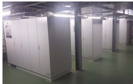
Figure 2: Power supplies (each 2.8 m x 0.8 m x 2m) installed in the basement.
