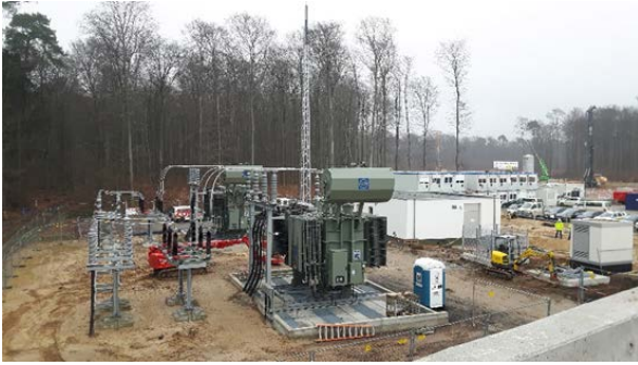
Figure 15: FAIR transformer field North
