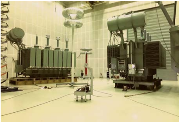
Figure 16: New Transformer in test field
