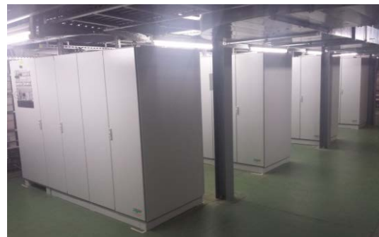
Figure 2: Power supplies (each 2.8 m x 0.8 m x 2m) installed in the basement.
