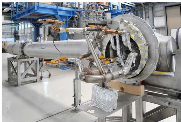
Figure 6: First-of-Series cryogenic bypass line of the local cryogenic system of SIS100 installed at the GSI Series Test Facility
