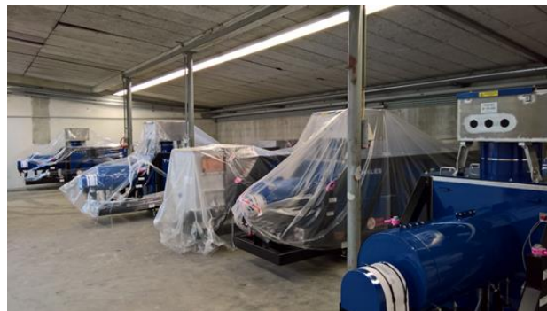
Figure 1: The Thales Klystrons #2-#7 are stored.
