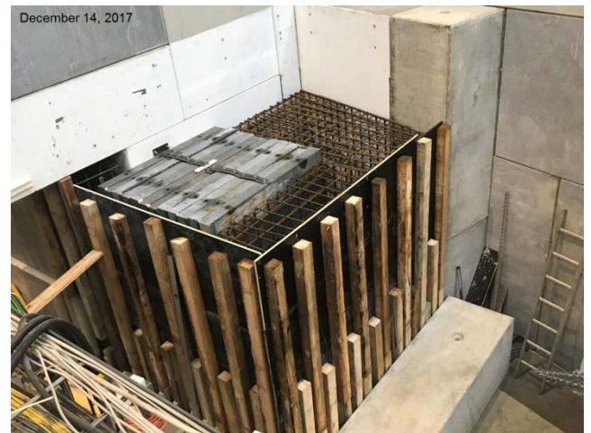
Figure 6: The Iron core of the beam dump is prepared for concrete pouring.
