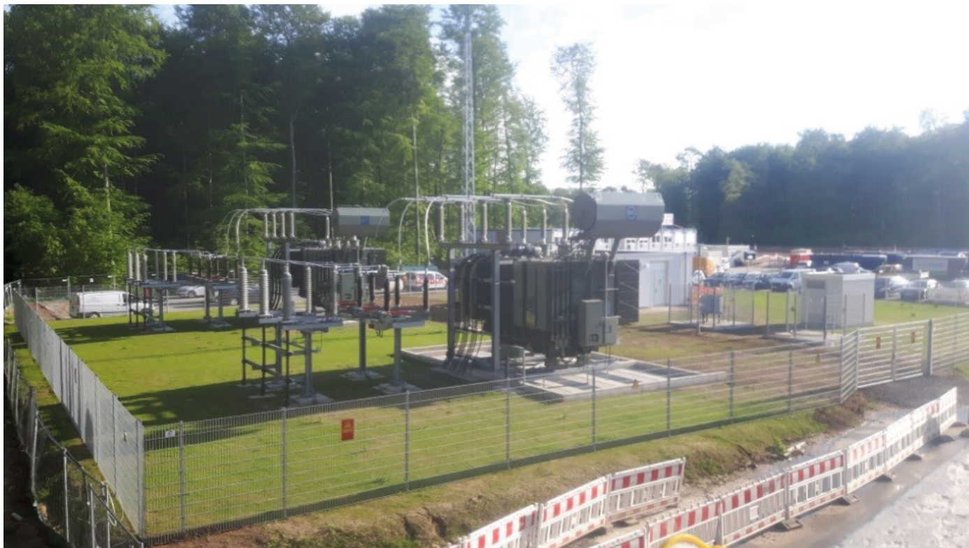
Figure 52. FAIR transformer station north
