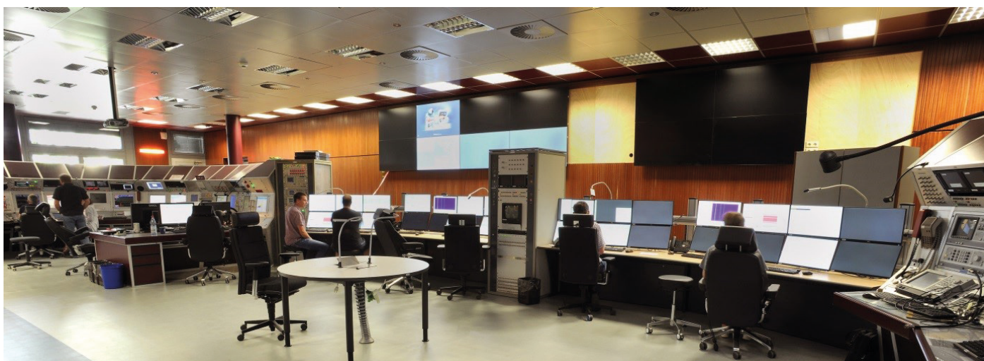
Figure 56. GSI control room refurbished with new FAIR consoles and fixed displays
