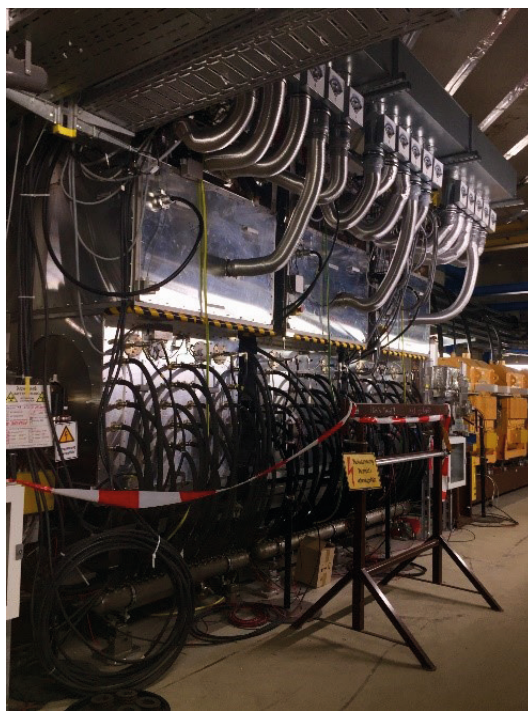
Figure 38. The three new MA loaded Rf acceleration cavities installed in SIS18. The cavity will allow acceleration of low charge state heavy ions (e.g. U^{28+} ) with maximum ramp rate.
