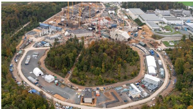
Figure 1: View on the FAIR construction site with the re-filled SIS100 tunnel pit in front.
