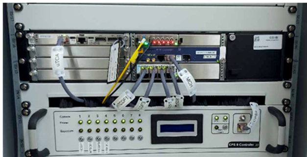
Figure 8: MTCA.4 DAQ system for GigE camera readout.
