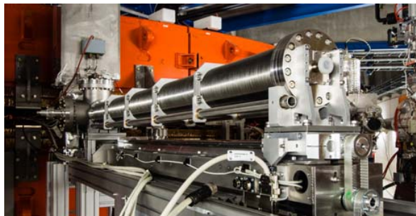
Figure 1: New detector manipulator in the first dipole magnet of the south arc (behind the electron cooler) of the ESR.
